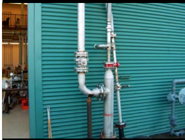
Outside connection to LFG
