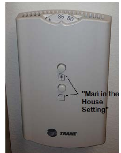
Figure 9. Thermostat in Building Site 4.
